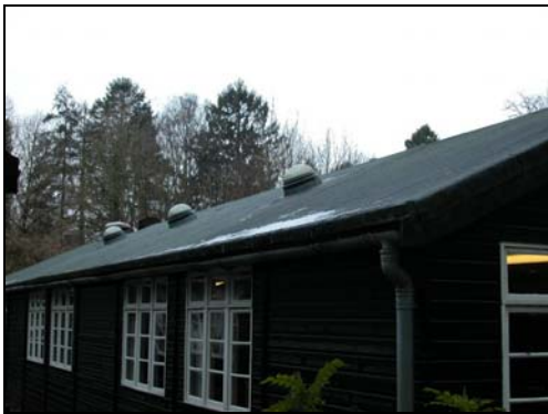
Fig 3: The Sun-Pipes from the Outside of the Building
